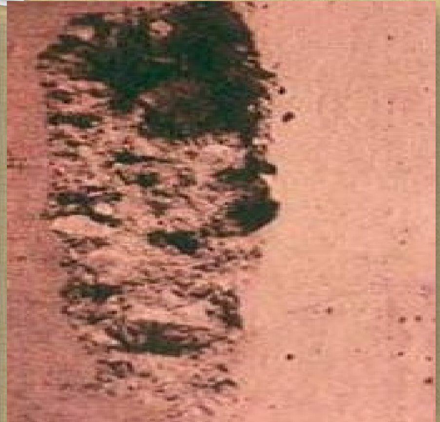
Sticking to forms damage caused during stripping of formwork from concrete.
