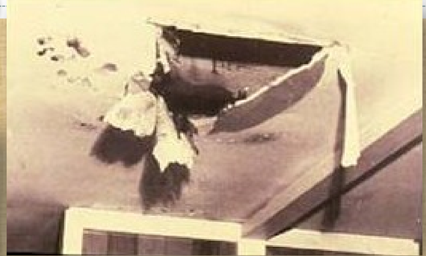
Dampness on ceiling-roofs leaks
