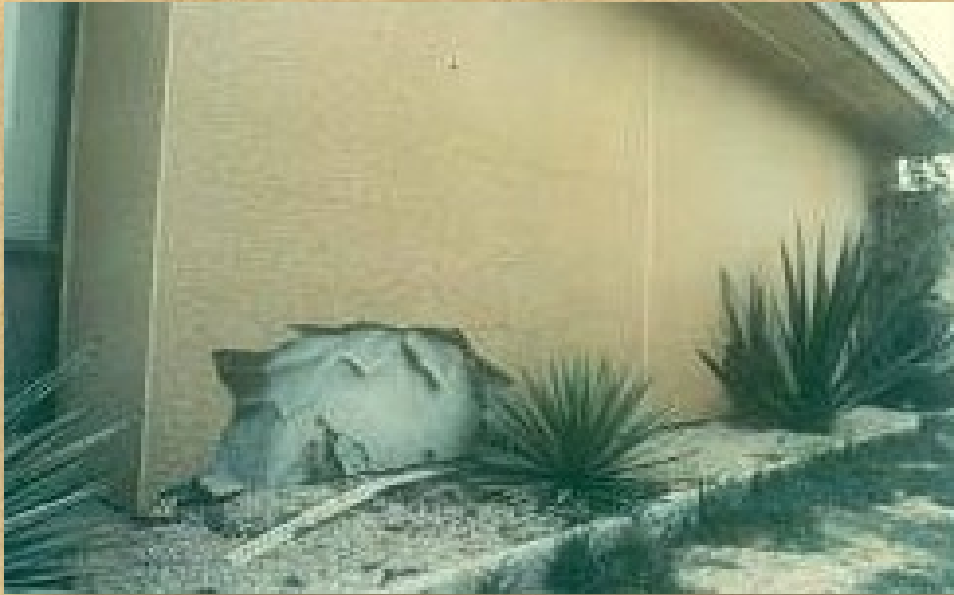
External finishing- presence of moisture in between
