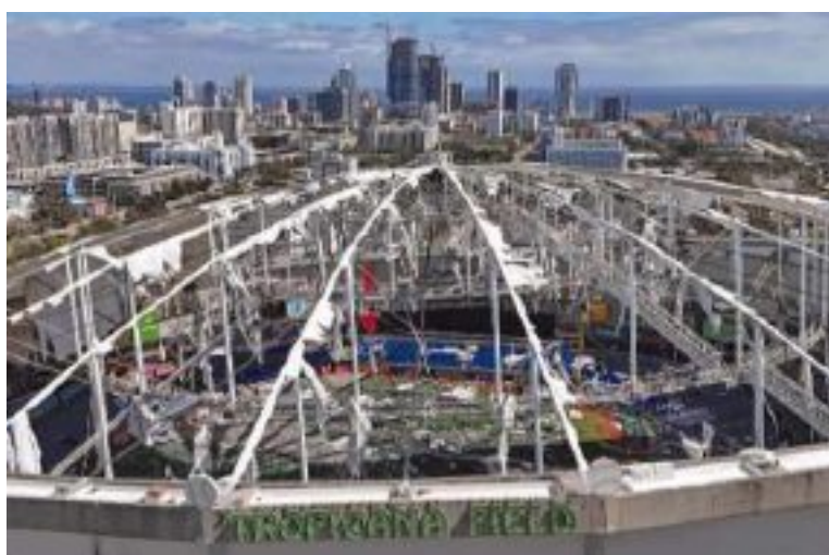
Above: the home ground of the Tampa Bay Rays baseball team in St Petersburg, Florida, lies in tatters a day after it was hit by Hurricane Milton in October
