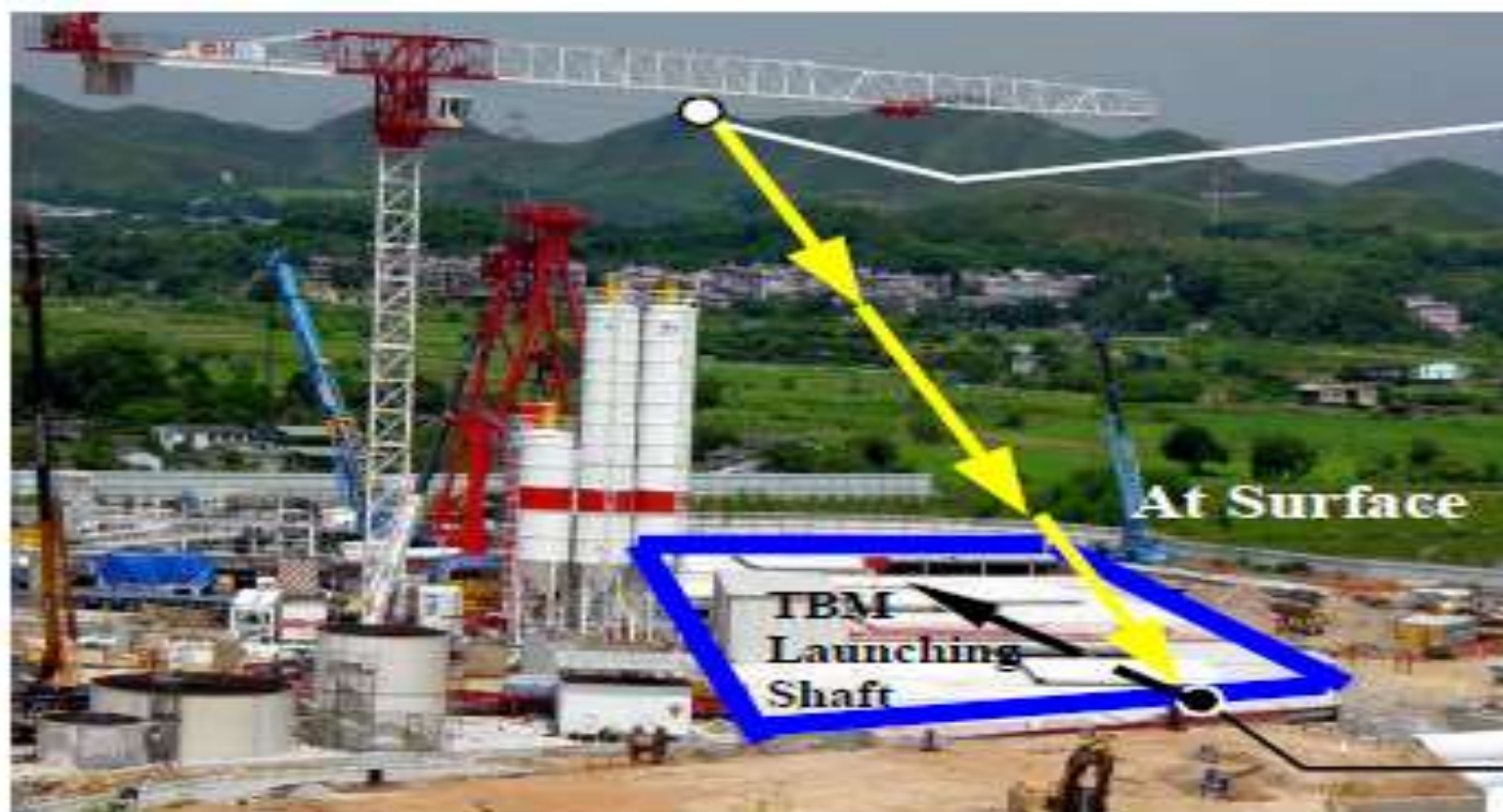
Figure 7 Transfer of control station at surface
