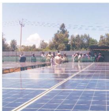
A solar power project at Kimbimbi, Kirinyaga County. [Munene Kamau, Standard]
