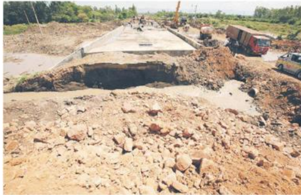
A section of Katito-Ahero road at Ayweyo that has cut off two towns, forcing motorists to drive for about 50km to reach Ahero, which ideally would have taken five minutes. [Denish Ochieng, Standard]
