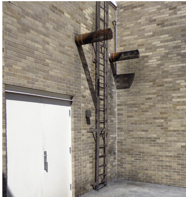
FIGURE 15.1 Unrestricted roof access.
