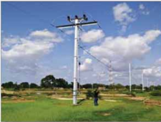
Electrification Project, Burkina Faso
