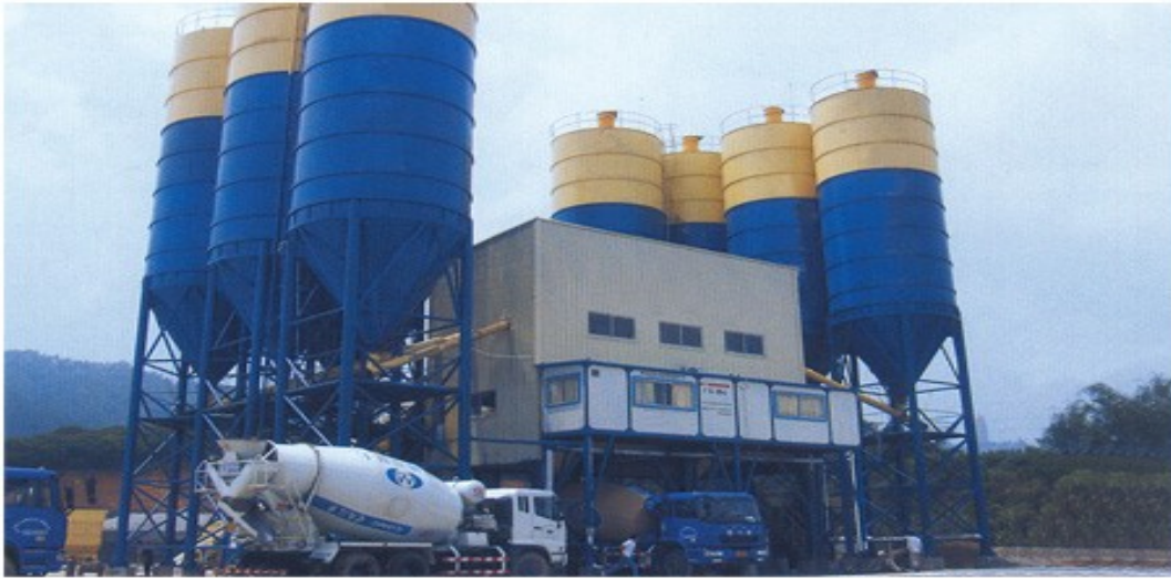
Gambar 9. 1 : Concrete Batching Plant.
