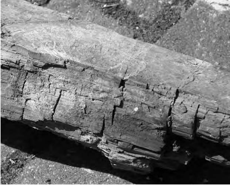
4.3 Brown rot in window frame edge. 4
