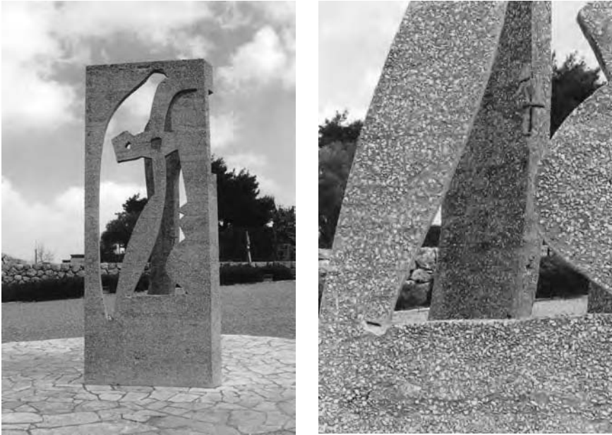
3.14 Reinforcement corrosion due to carbonation in concrete sculpture by Picasso (1967) in National Museum of Israel, Jerusalem.
