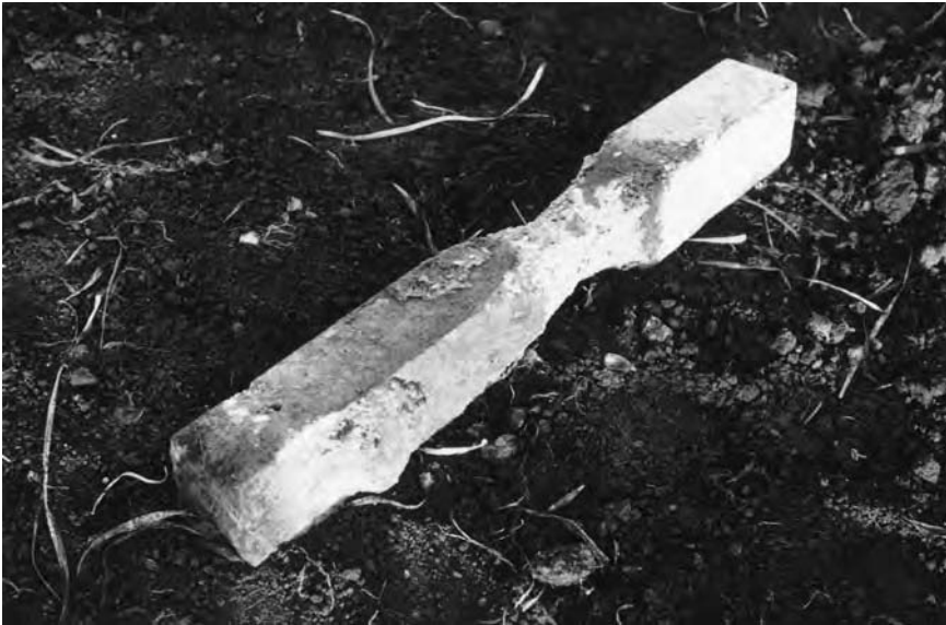
3.3 Deteriorated greenhouse foundation pile. 1
