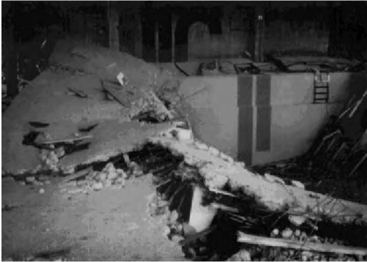
2.33 Concrete ceiling that collapsed in a swimming pool due to chloride-induced stress corrosion of stainless steel hanging strips in Uster, Switzerland, 1985.
