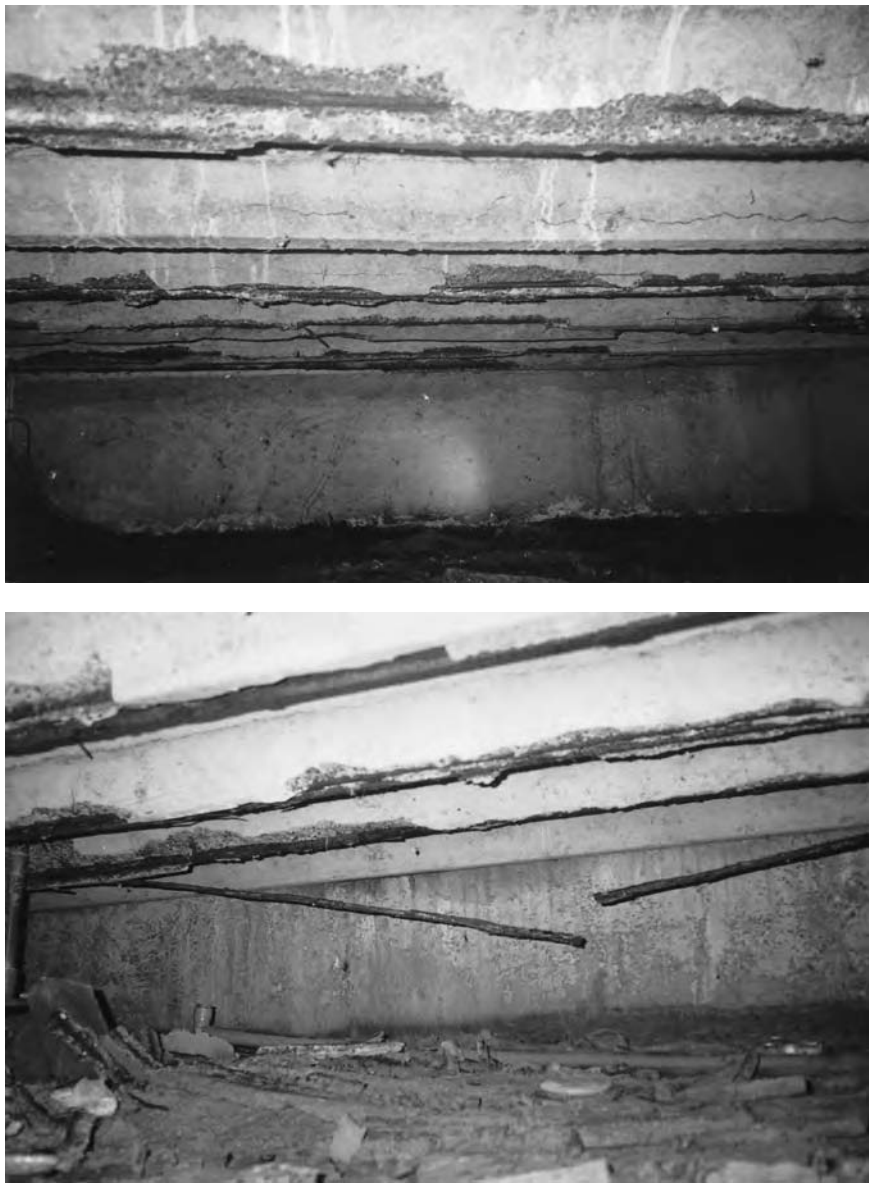
7.4 Photographs of damage of Kwaaitaal floors in crawl space.
