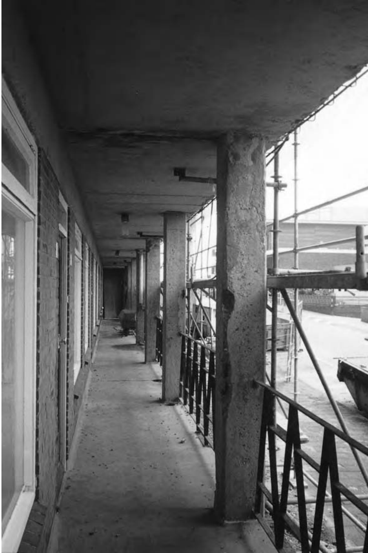
3.46 Local patch repair with adjacent new reinforcement corrosion.
